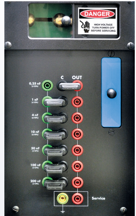
Capacitor selector switchboard
